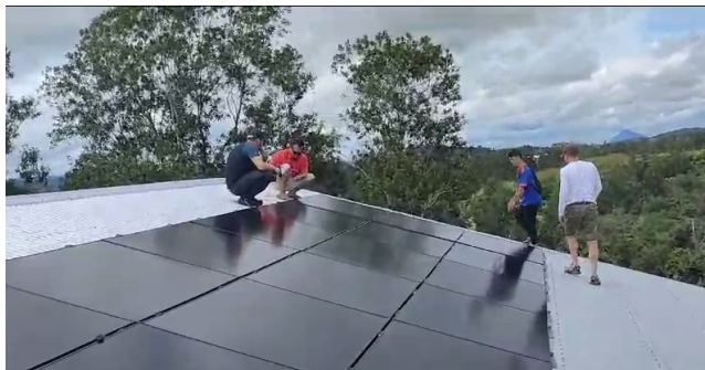
Our very first solar panels which gives Titus house electricity 24/7. What a blessing.
