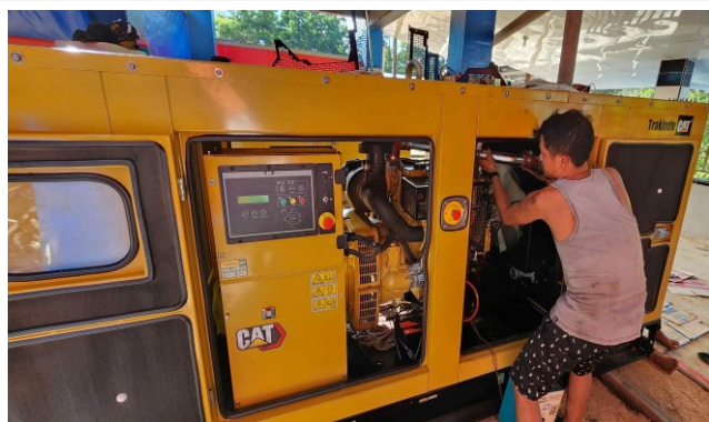
Our Samuel doing a wonderful job servicing one of our many generators that constantly require maintenance and upkeep. It's a huge responsibility for him and his team.
