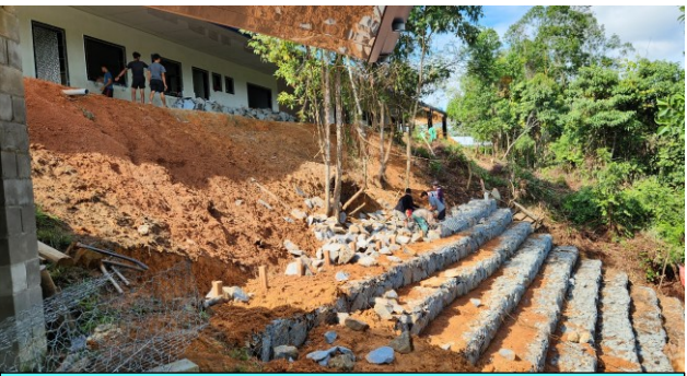
A lot of erosion prevention to be built for almost every building we erect.
