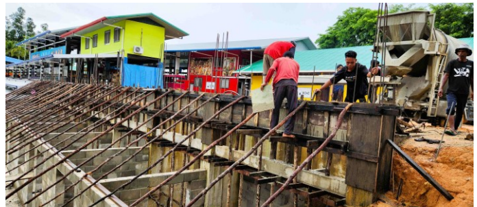
Four homes being built for couples who are trained to become house-parents. On top will be 2 floors of storage area.
