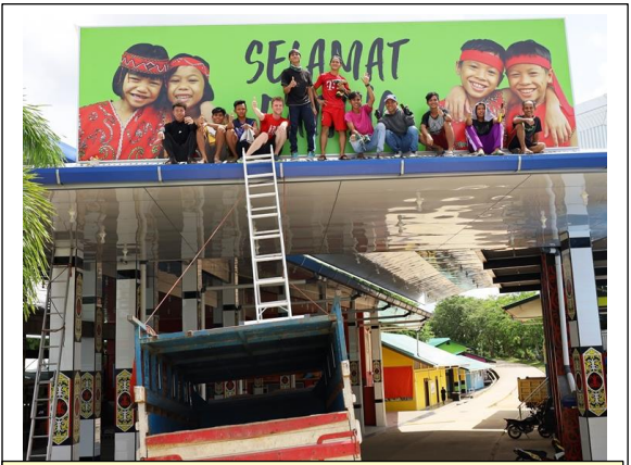
One of our fabulous work teams erecting the huge sign at the entrance of our training centre, Borneo style.
