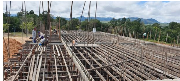
Preparations for a concrete slab for the second floor of the new 12 classroom school building.
