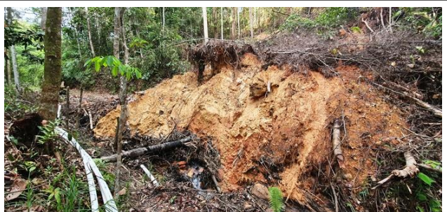
Our road to our dam cut off due to quite a long landslide.
