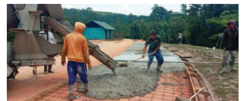
Concreting our roads, so no more dangerous mishaps during rain-season and no more expensive repairs.
