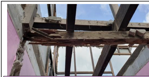
White ants have been busy destroying our home.
